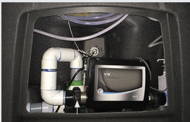
FIGURE 1.9a : HEATER UNION; LOOSEN UP TO BLEED AIR
